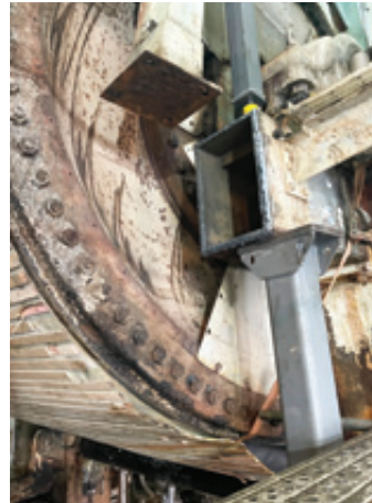
Yankee surface protected, head insulation panels removed, temporary support structure in place and beam flame cut and prepared
